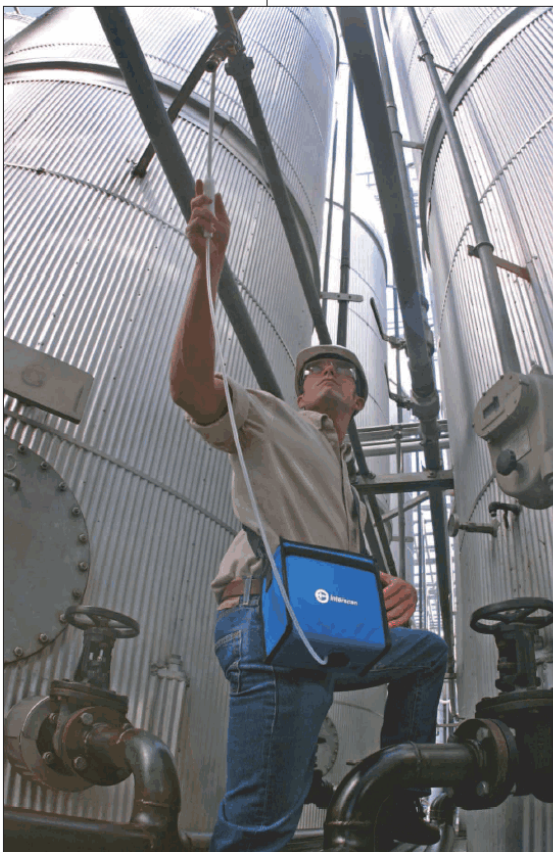
Checking a solenoid valve in a formalin line.
